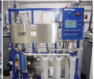
Water Filtration System
