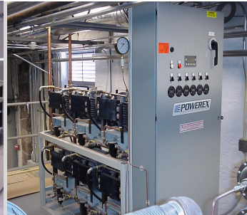
Vacuum Pump System
